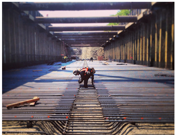
Workers Construct the BART Phase I Extension to Berryessa Image courtesy of VTA
